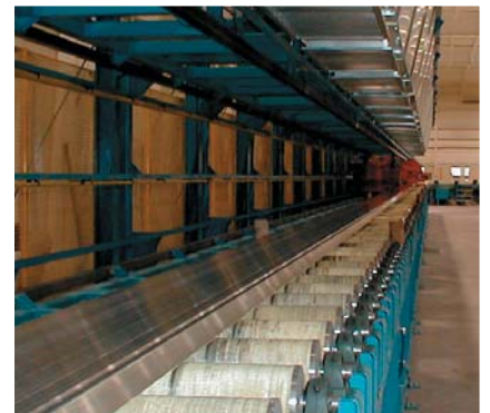
Runout roller conveyor and overhead air cooling system
